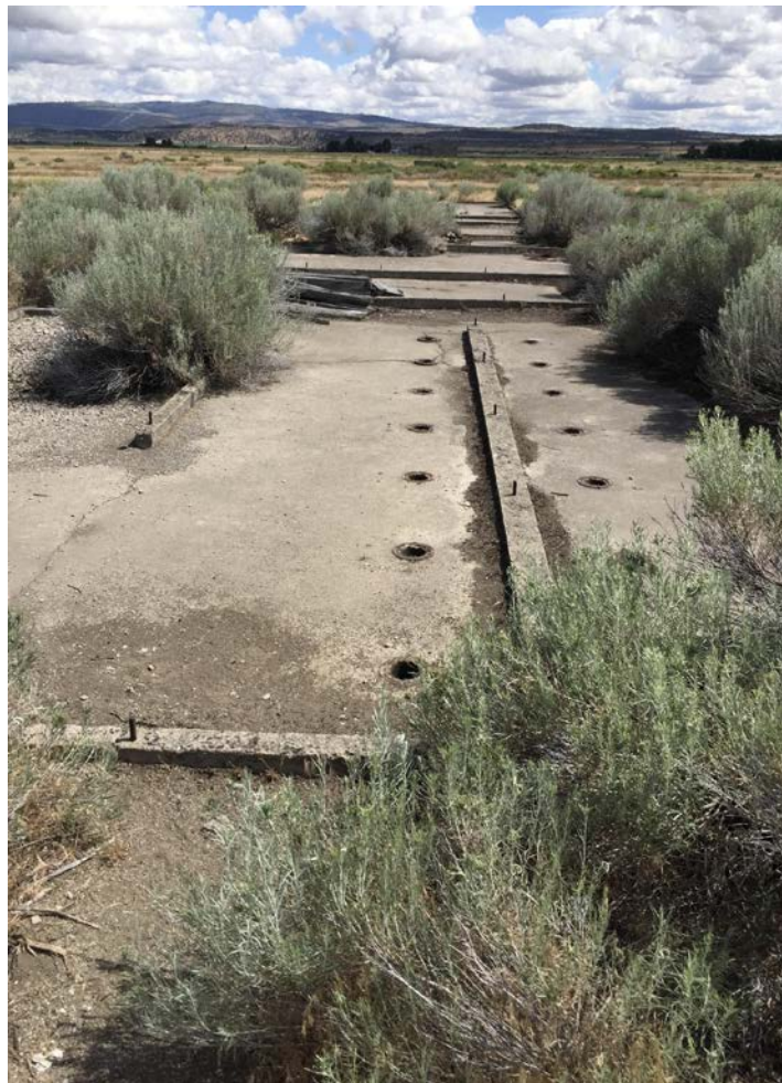
Foundation of a Tule Lake Bathhouse with Latrine [Maureen Burns photograph, July 9, 2016]
